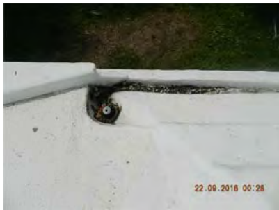
Debris at downspouts. Clean and maintain
