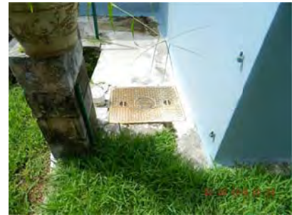
Clean out access lid
