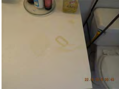
Bathroom vanity top staining
