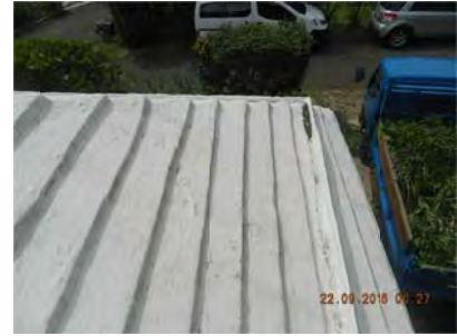
Roof shows some flaking and spalling. Some debris accumulation in gutter glides.
