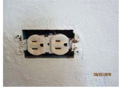
4.18 Receptacle outlet appeared generally sound.
