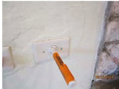
4.23 220V Receptacle here had no power. North wall area.
