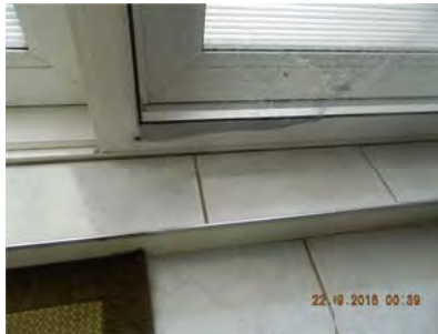
South door screen needs repair
