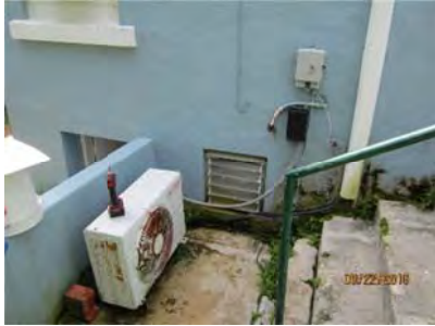
6.7 A Split system condensing unit located on the east side of dwelling is not functional.
