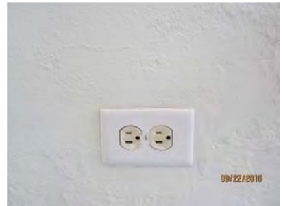
1.15 Receptacle outlet appeared generally sound.
