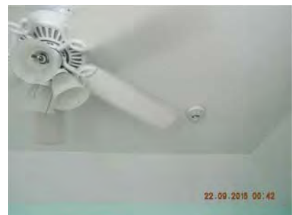
Smoke detectors disconnected.
