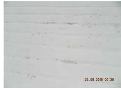
Flaking and general deterioration of roof coating(s)
