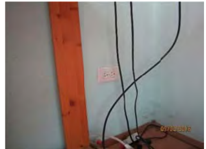
4.30 Receptacle outlet appeared generally sound.
