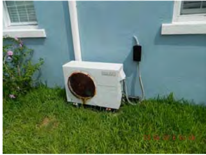
AC unit not tested but shows some corrosion
