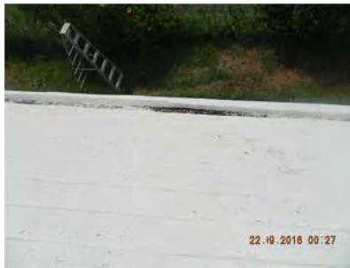
Water ponding at mold staining
