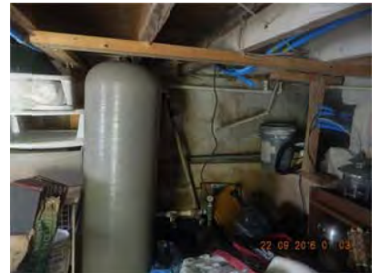
Pre-pressurized tank is functional and satisfactory
