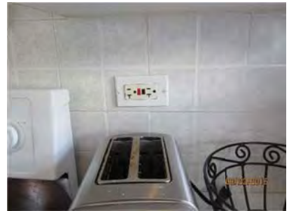
4.3 GFCI north wall tested ok.
