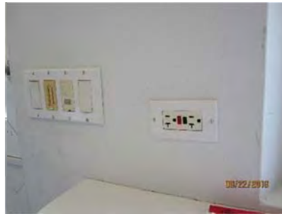
4.2 GFCI east wall tested ok.
