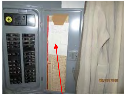
3.6 The panel directory needs to be completed.
