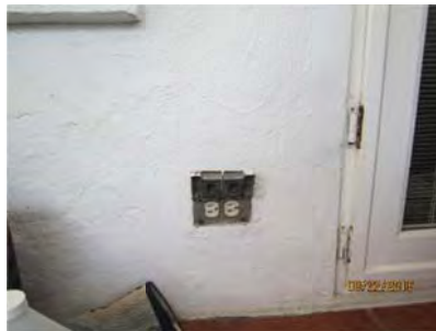
6.5 Receptacle outlet located on the south porch needs a GFCI receptacle installed to protect personnel from electrical shocks.
