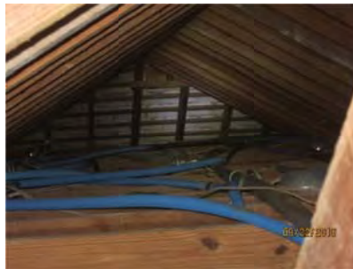
4.59 A blank plate is need for the J box above living room area.
