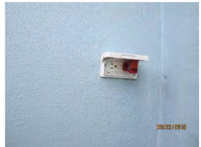
6.6 GFCI receptacle located east side of dwelling tested ok. Appeared generally sound.
