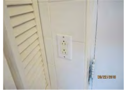
4.45 GFCI Receptacle outlet tested ok. Appeared generally sound.
