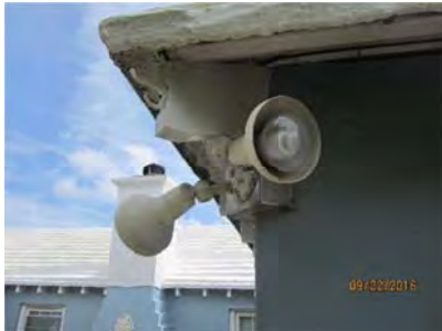
6.1 Exterior fixture north corner did not function. Needs new bulbs.
