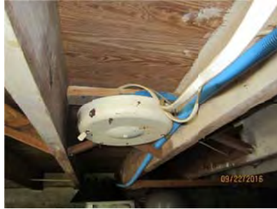
5.3 Fixture did not function and needs to be replaced.
