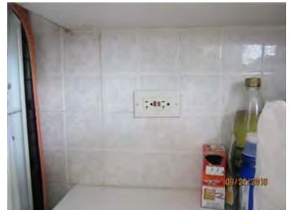
4.6 GFCI south wall tested ok.
