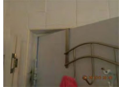
Bathroom door binds.
