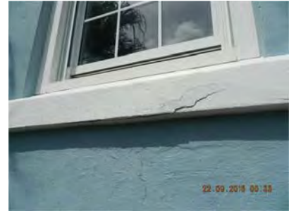
Possible rebar spalling at window brow
