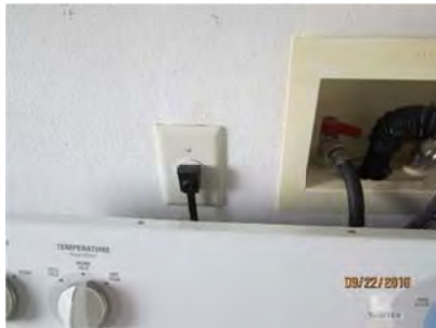
4.10 Washer and receptacle outlet appeared generally sound.
