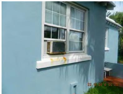
Rust staining from window AC
