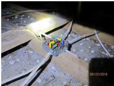
4.58 A blank plate is needed for the J box (east bedroom closet access).
