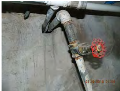
Older galvanized pressure lines and valves
