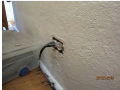
4.41 Receptacle outlet appeared generally sound but a cover plate is needed.
