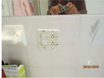
4.44 GFCI Receptacle outlet tested ok. Appeared generally sound.
