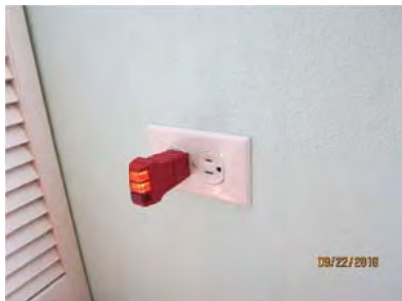
4.31 Receptacle outlet appeared generally sound.
