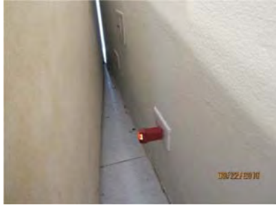
4.25 Receptacle outlet appeared generally sound.
