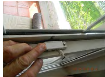
Several window latches need adjustment/repair
