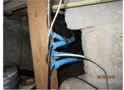
5.4 BTC and CV cables, conduits need tidying.
