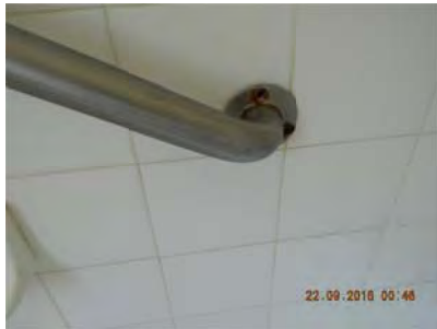
Shower grab bar screws are corroded
