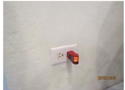
4.24 Receptacle outlet appeared generally sound
