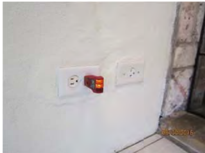
4.22 Receptacle outlet appeared generally sound.
