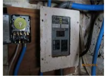
2.1 A 12-CCT 120/240V Main distribution panel is located in the basement. The panel directory needs to be filled.
