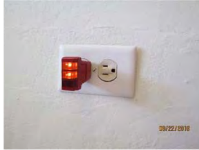
4.17 Receptacle outlet appeared generally sound.
