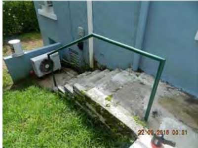
Steps and railing with outdoor AC
