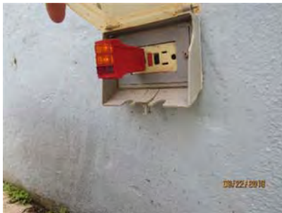
6.4 A GFCI receptacle located outside kitchen door area tested ok. Appears generally sound but needs a new weather proof cover.
