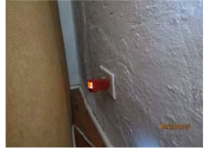
4.54 Receptacle outlet appeared generally sound.
