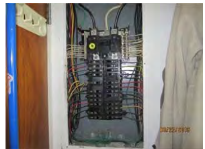
3.4 Circuit breakers, conductors and feeder appear generally sound. 220V Circuits 9/11 have been disconnected
