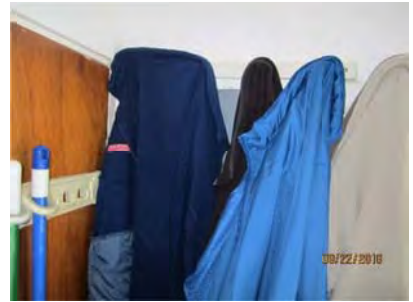
3.7 Panel located behind these jackets.
