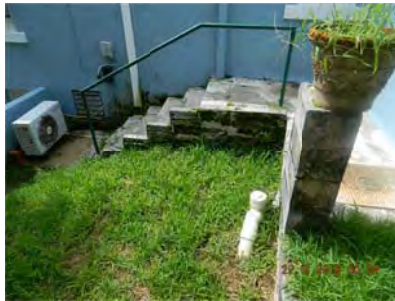
Stair railing is functional but not code compliant
