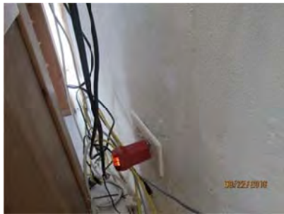
4.19 Receptacle outlet appeared generally sound.
