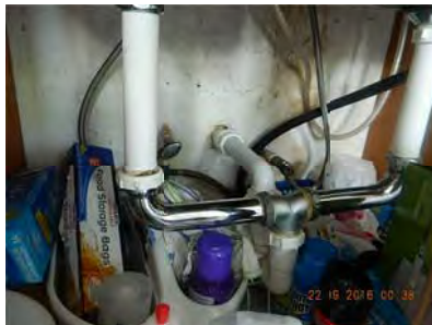
Belwo sink plumbing
