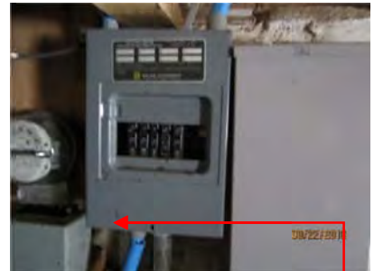
3.1 A 8-CCT 120/240V Sub panel located in the basement. Appears generally sound. Screw for cover needs to be installed.
