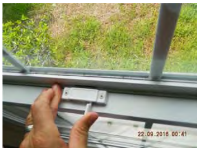
Defective window latch
