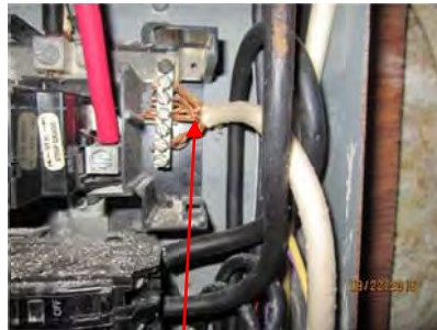
2.3 The neutral conductor must terminate on a single lug. Lug needs to be installed.
