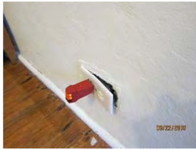
4.38 Receptacle's tab has rusted out, device needs replacing.
