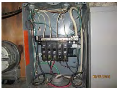
3.2 Circuit breakers, conductors and feeder appear generally sound.
