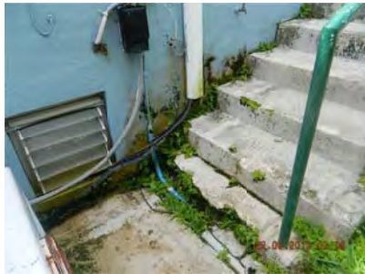
Step needs repair. Remove vegetation
