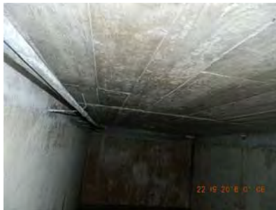
Tank view looking east. Note galvanized suction line
