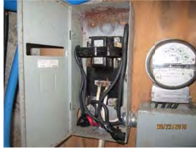
1.2 Disconnect not in use as a switch but now used as a junction box.
