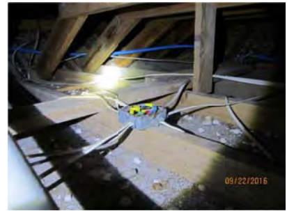
4.57 Roof Space NM cable, mostly the wiring method of choice, appears generally sound.
