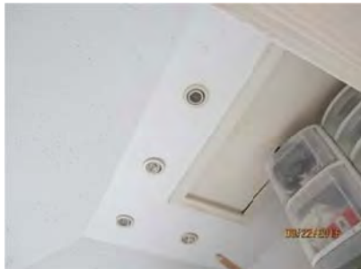
4.13 The ceilings lights in the laundry did not function. Likely bulbs need changing.
