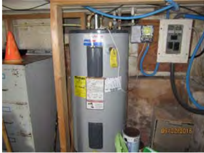
5.2 A Domestic Water heater is located in basement. The time clock, circuit appeared generally sound.
