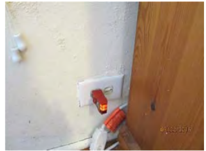
4.39 Receptacle outlet appeared generally sound.
