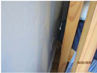
4.55 Receptacle outlet appeared generally sound.
