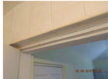
Bathroom door needs adjustment
