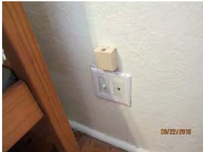
4.40 Receptacle outlet appeared generally sound.
