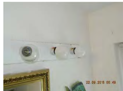
Light fixture shows some rust
