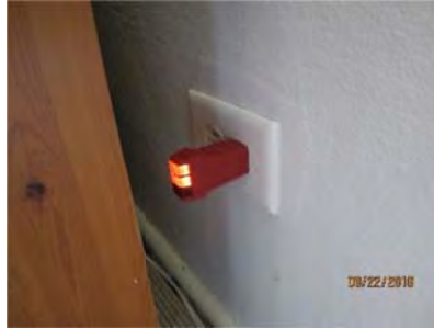
4.53 Receptacle outlet appeared generally sound.
