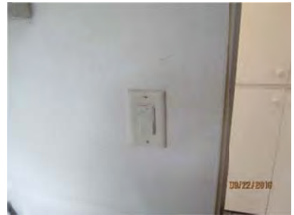
4.12 Switch for laundry room lights appeared generally sound.
