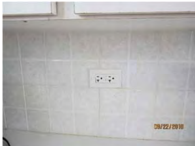
4.4 GFCI north wall tested ok.
