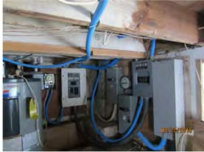
1.1 A Single 100A 120/240V single-phase metered service located within the basement east side of dwelling. Appears general sound.
