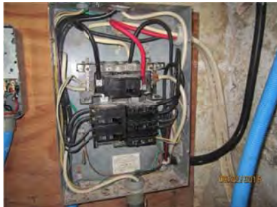
2.2 Circuit breakers, conductors and feeder appear generally sound.
