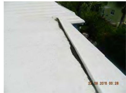
Porch roof gutter glide, water ponding
