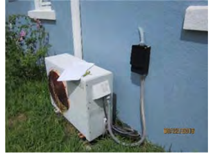
6.9 A Split system condensing unit located on the west side of dwelling is not functional.
