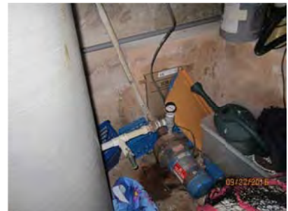
5.1 Pump/Utility room/Water heater located in the basement. Fixtures switches and outlets appeared generally sound.
