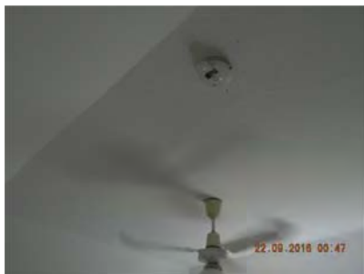
Smoke detector disconnected
