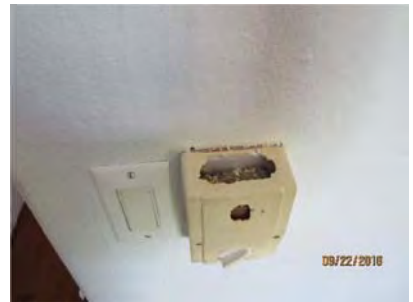
4.51 Fan control is deteriorated, need replacing.
