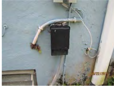
6.8 Disconnects for the condensing units were disconnected.
